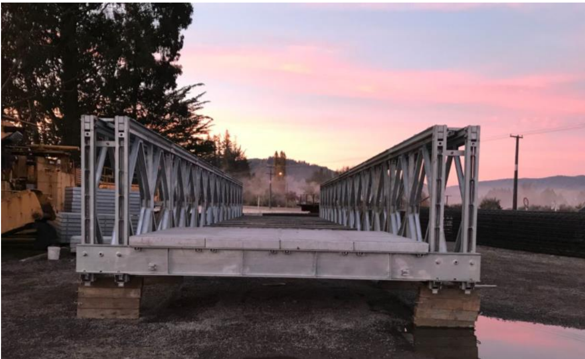
The Bridge which will provide all weather access to the project site has been constructed by the team at Reefton Cranes ahead of installation at site in October.
